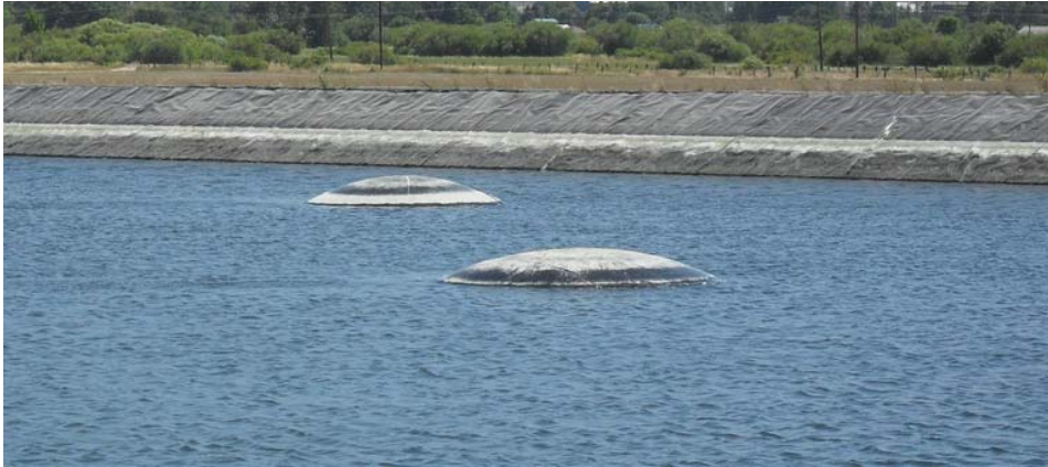
Figure 1. Bubbles in pond with 1.5 mm HDPE geomembrane on verge of bursting.
